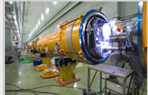
Crew welding the pipes at the far upstream end of the cryostat (TESLA-type cavity part).
