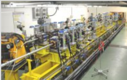
A view of the two beam lines in the CLIC experimental hall.
