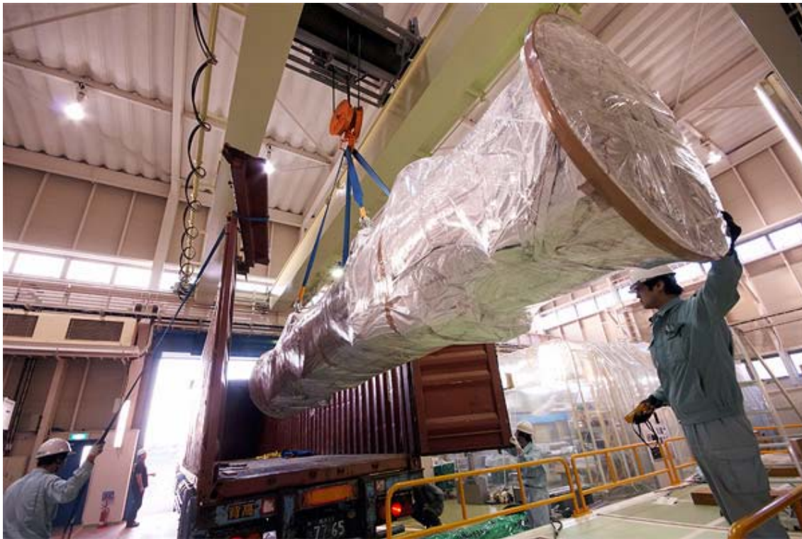
Italian made cryomodule being taken out from the container at Superconducting radiofrequency Test Facility (STF) at KEK.
