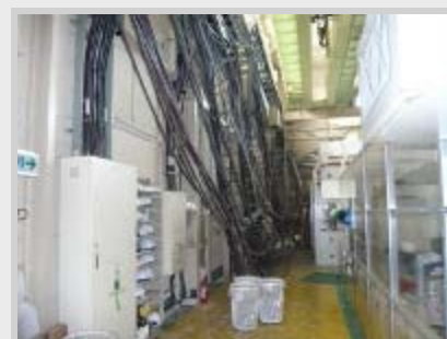
The primary damage to ATF, with fallen cable racks and cables. It will require about a month to repair.
