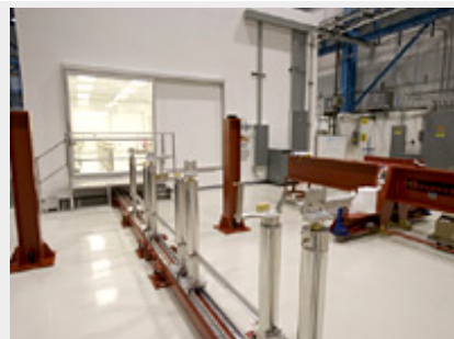
A rail system runs under the entire clean room, where the cavities rest and await assembly.
