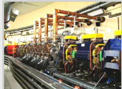
Indus-II Accelerator at Raja Ramanna Center of Advanced Technologies (In View RF Cavities).
