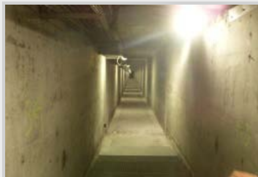
The path to safety. This oxygenated escape tunnel is accessible from the road level above it through a safety shelter. It runs the entire length of the Mont Blanc tunnel, 11.6 kilometres. Image: John Osborne
